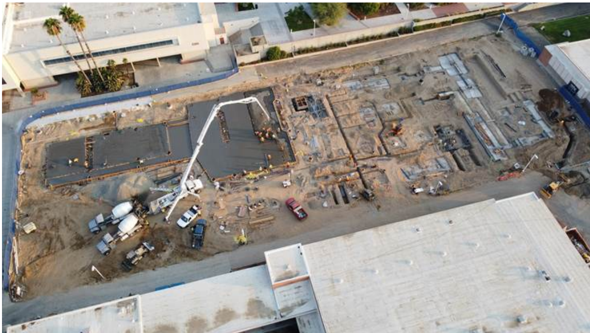
The cement slabs are down for our new Science and Engineering Building. #ABetterBC
