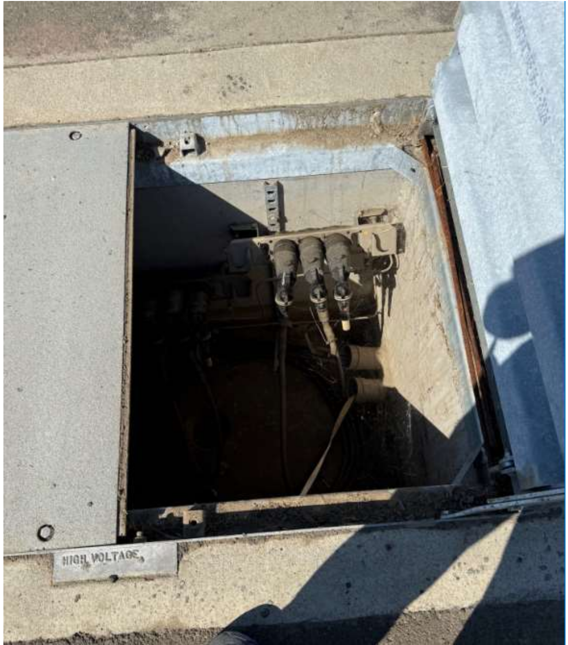
Figure 1: interior of electrical vault
