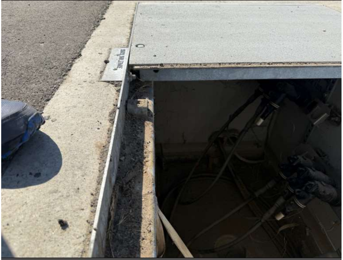
Figure 2: interior of electrical vault
