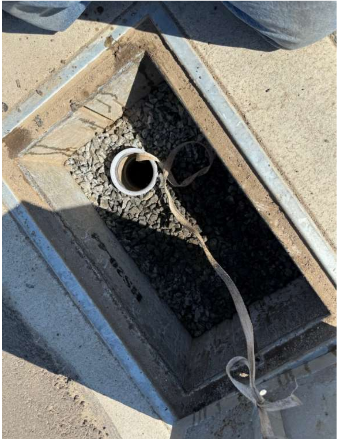
Figure 3: interior of small electrical vault
